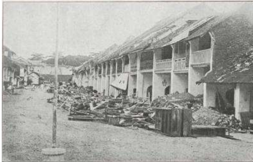
Figure 6: The condition of the Malabero Chinese shop house after the 1914 Bencoelen earthquake.
