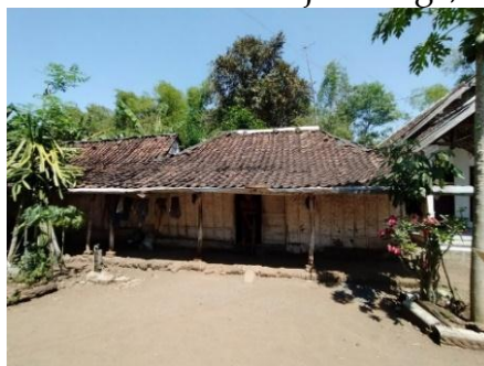
Figure 9. Condition of houses in Sumberejo Village, Pandaan District in 2023
